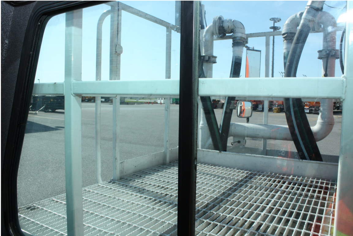
Figure 8. View from inside an identical tanker, looking through the right-hand window with the service platform stowed (Source: TSB)
